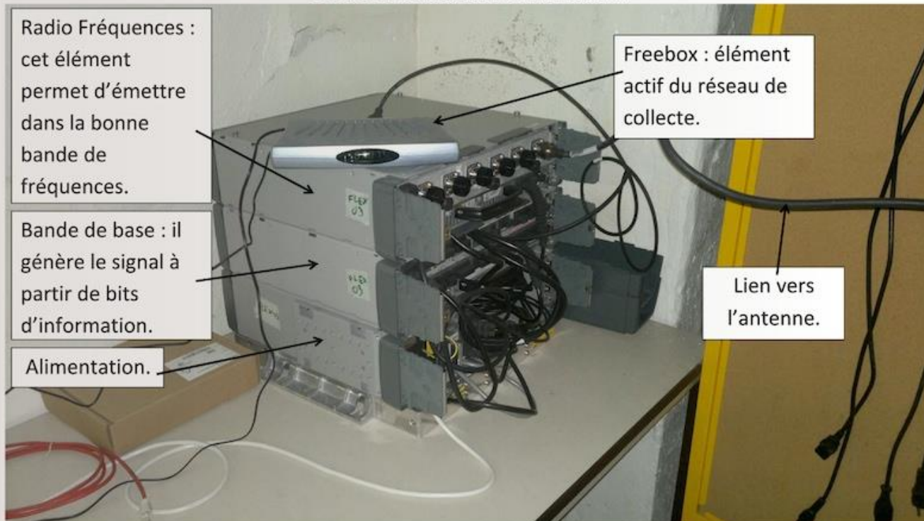
Station de base Free Mobile
